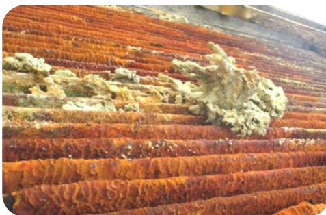
Corroded metallic air preheater
